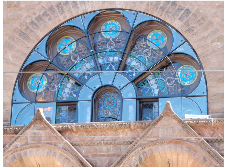
DURING: Details of the stained glass are so well seen during the replacement process.
