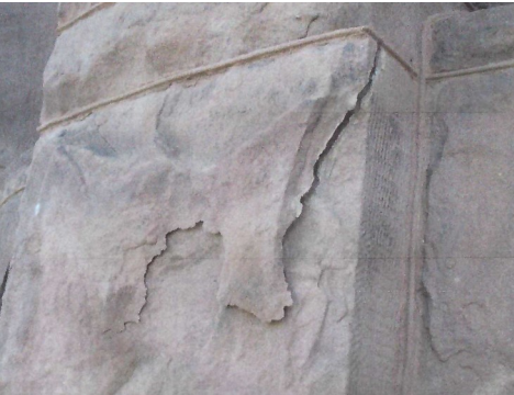
BEFORE: Stone surface cracking, on the verge of breaking.
