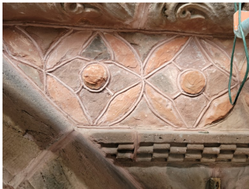
AFTER: Deteriorating patches were replaced, retaining as much of the original stone as possible.
