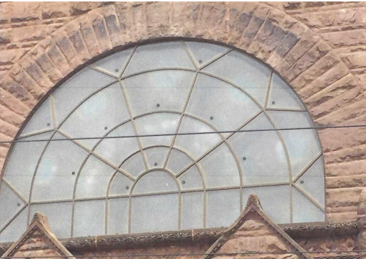
BEFORE: Storm window covers were cloudy over the stained glass window, concealing the wood frame.
