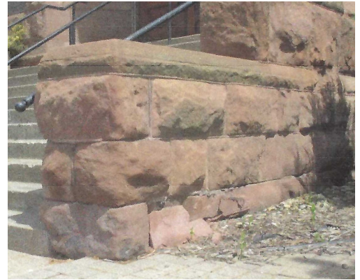
BEFORE: Spalled (fractured) and crumbling stone and mortar joints on stair wall by entry.
