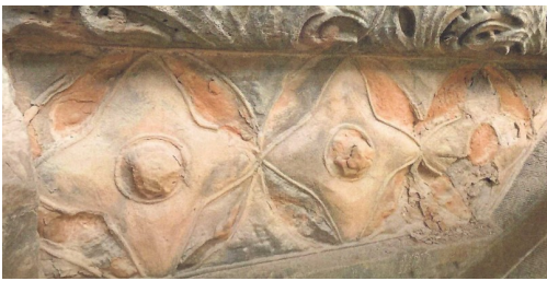
BEFORE: Previous patchwork of rosettes above main entrance were deteriorating.
